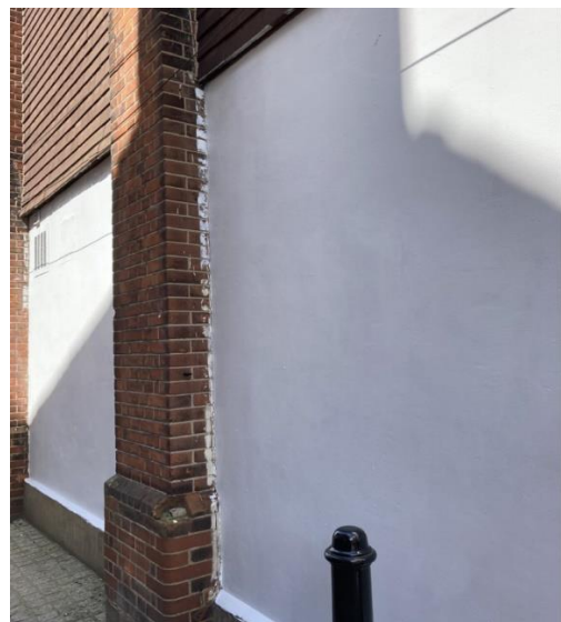
Photo after graffiti removed (June 2024)
